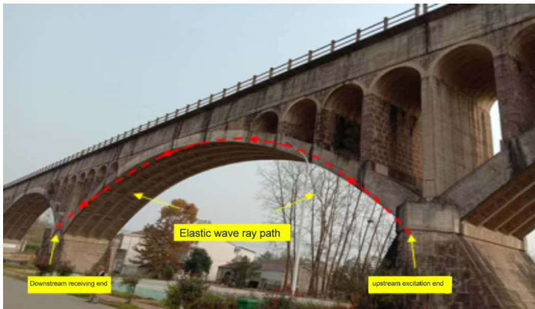
Figure 1. Overall Concrete Quality of the Arch Ring Beams Detected by Impact Elastic Wave Testing
