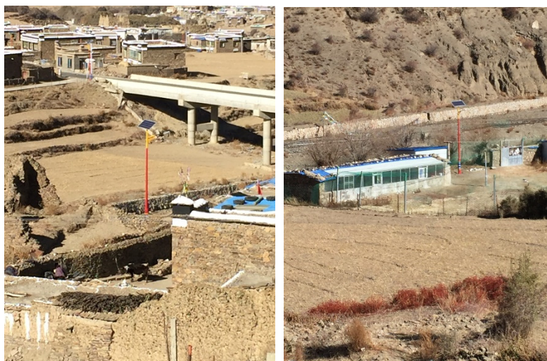
Fig 2. Acceptance Photo of Solar LED Street Lamp
