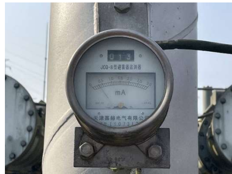
(b) Surge arrester leakage current monitoring instrument
