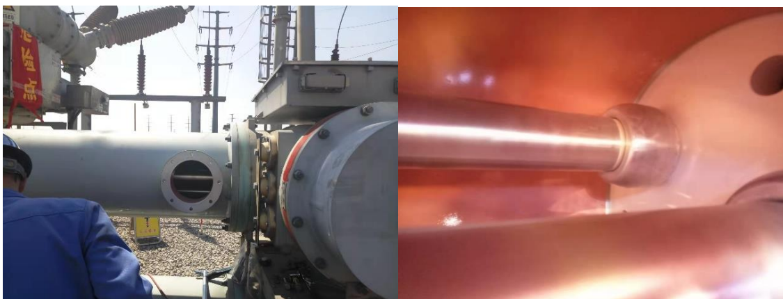
Figure 1. GIS internal defects
