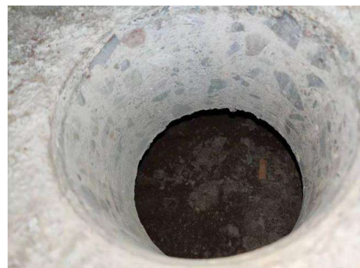
Figure.2 Sinking of the atrium backfill
