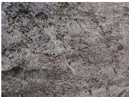
Figure.1 Cracking of the surface
