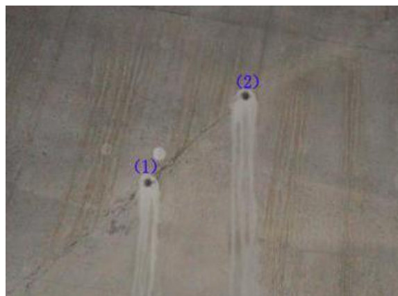
Figure 4. second lining crack drilling position
