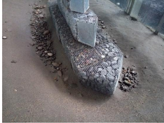
Fig3 Front end triangle basis protecting bridge pier
