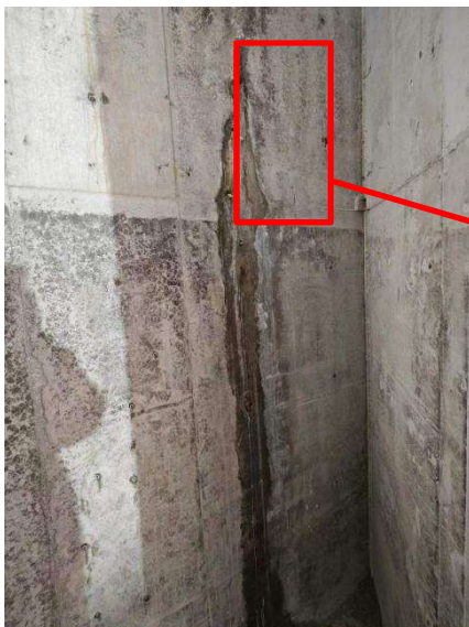
Figure 1. Water seepage on the wall
