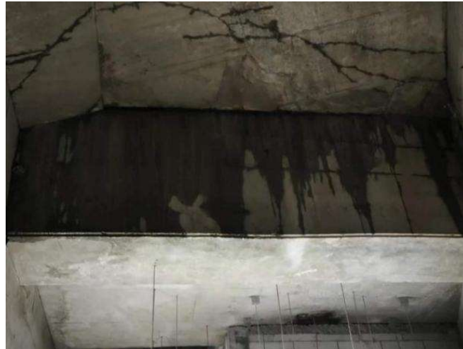
Figure 3. Water seepage in the joint of the structure
