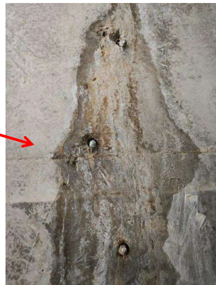
Figure 2. Water seepage at the water stop needle
